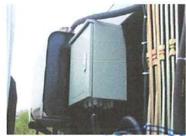
PLC Modular control box
